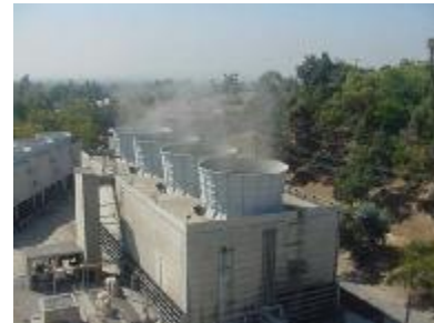
Cooling towers using steam for heat rejection.
