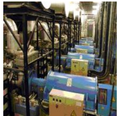
21 st century fly-wheel generators
